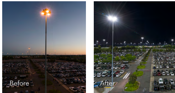
Sacramento Airport improved visibility and reduced energy costs by replacing HID high mast lighting with HMLED2 fixtures from Holophane®.
